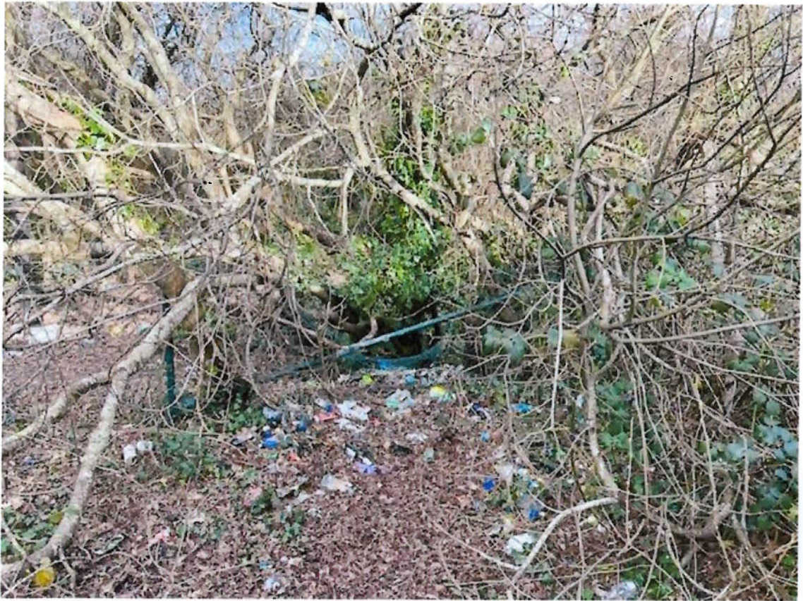
Figure 3: Former chain link fence (which has now been replaced) and unauthorised rubbish/fly tipping
