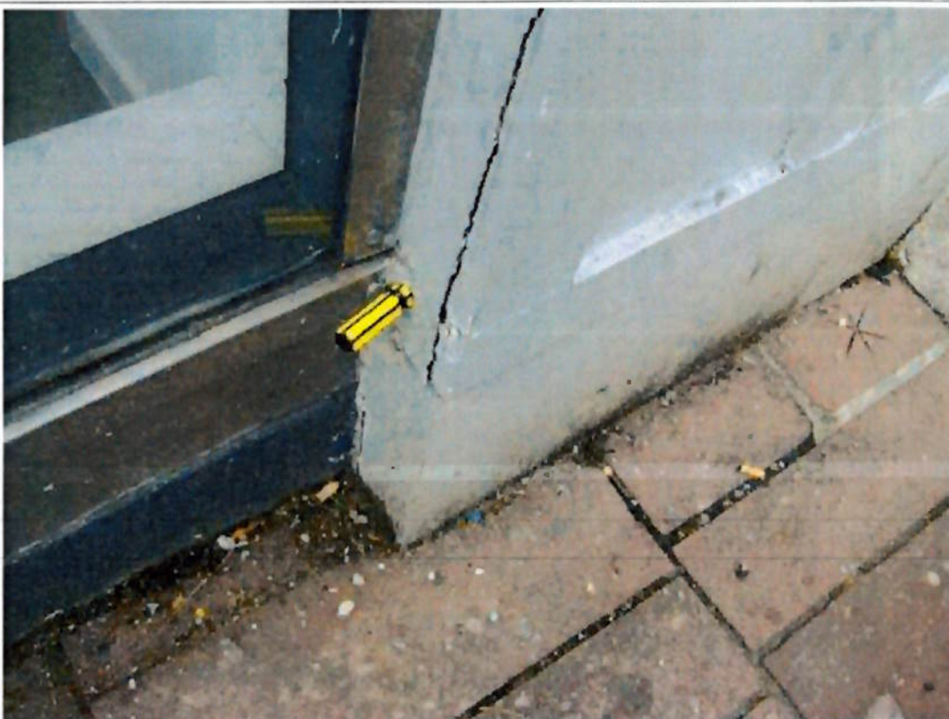
Photograph 24 View of screwdriver puncturing through decayed timber.
