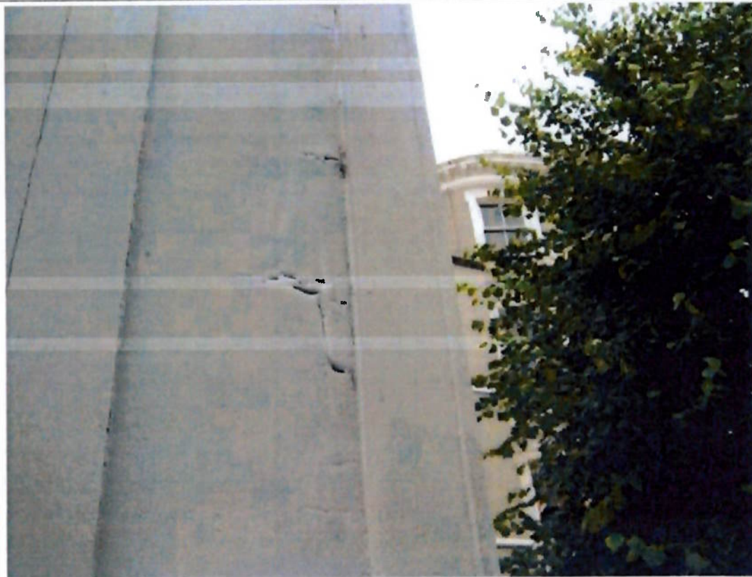
Photograph 21 View of blistering paint to Column 2.
