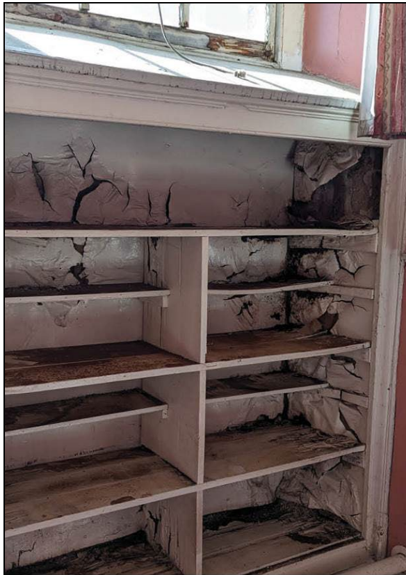
Detail of window and cupboard to south of Room F08 showing damage.
