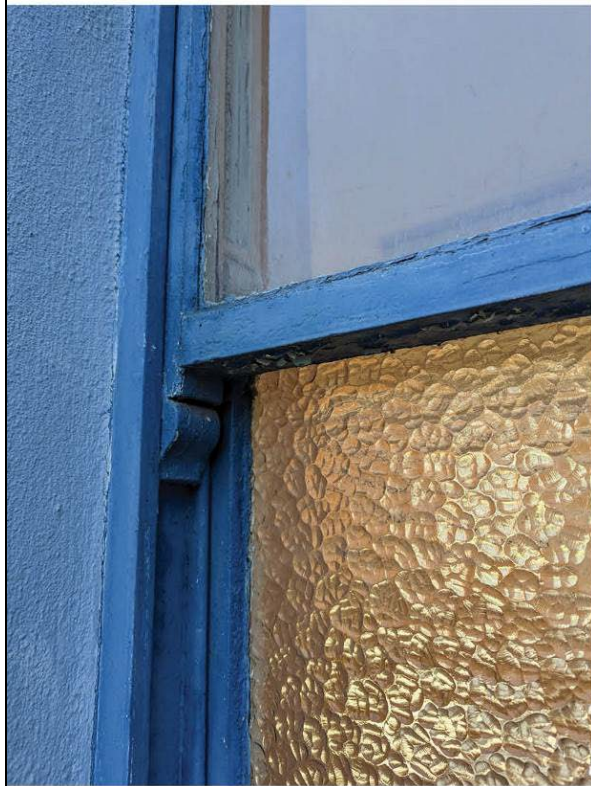
Detail of sash on window to G04.
