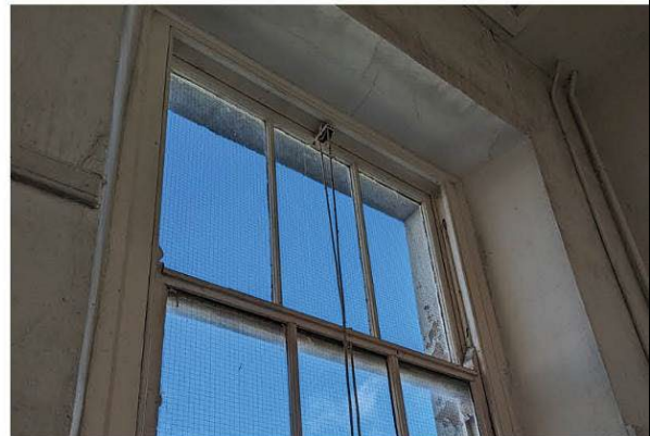
Detail of window in F01 showing replacement wired glass.
