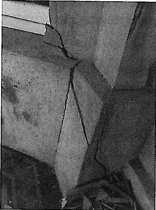
Photo 22 – Movement in South West Corner Bay
