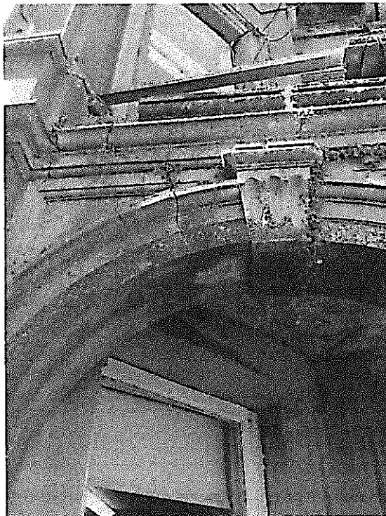
Photo 18 – Cracking in Arch
