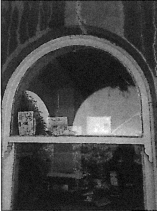
Photo 28 – Cracks around window
