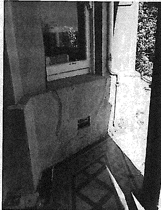
Photo 23 – Cracking in South East Corner Bay
