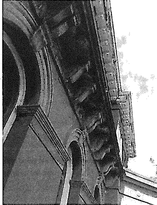
Photo 29 – Deterioration of Corncing
