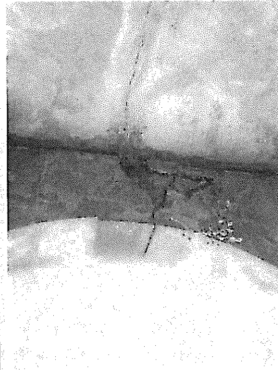
Photo 19 – Cracking in Arch
