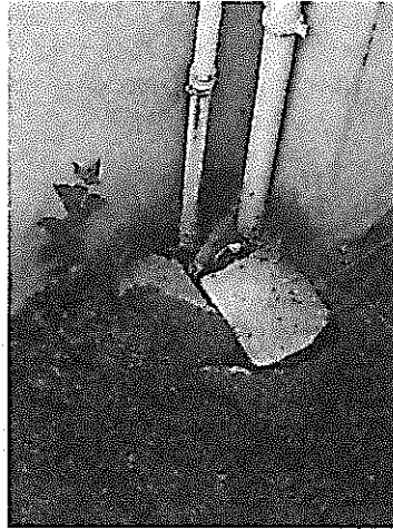
Photo -04 Gully in Well at Front Elevation
