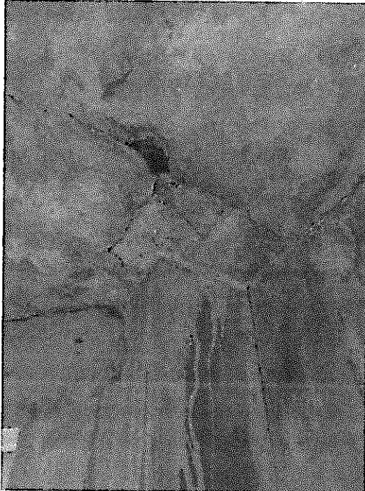
Photo 20 – Cracking to U/S of Concrete Walkway
