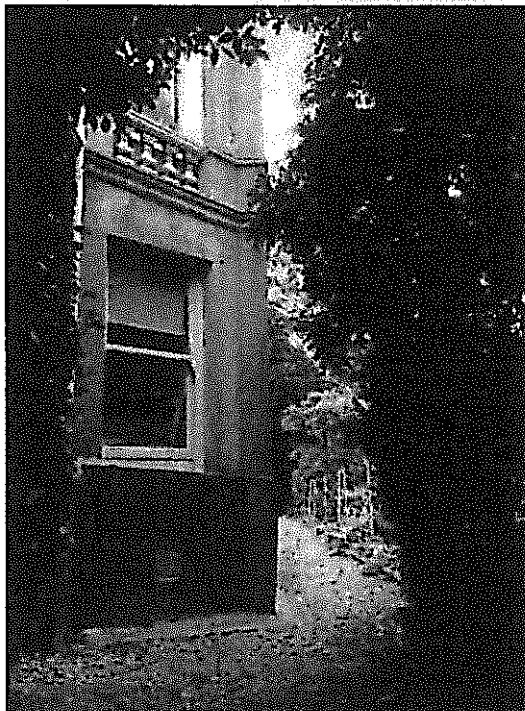
Photo 30 – South west bay window showing significant structural movment.
