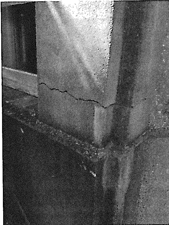
Photo 26 – Cracking in Walls
